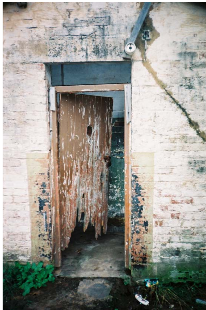
This picture shows the condition of this toilet. About fifteen people use this toilet, July 2005 (Photo by Sizwe Nzama, Durban South Photography Project).
